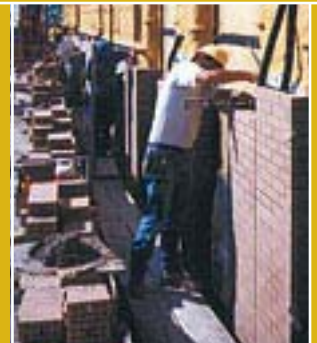
Ergonomic! The upper deck keeps the material at the right height for the workers standing on the lower step working area!
