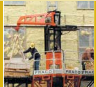
The optional Hydraulic Portable Crane FRH-2500 can bring material weighing up to 1,140 kg (2,500 lbs.) to the platform at a height of 100 m (330 ft) while workers continue with their jobs.
